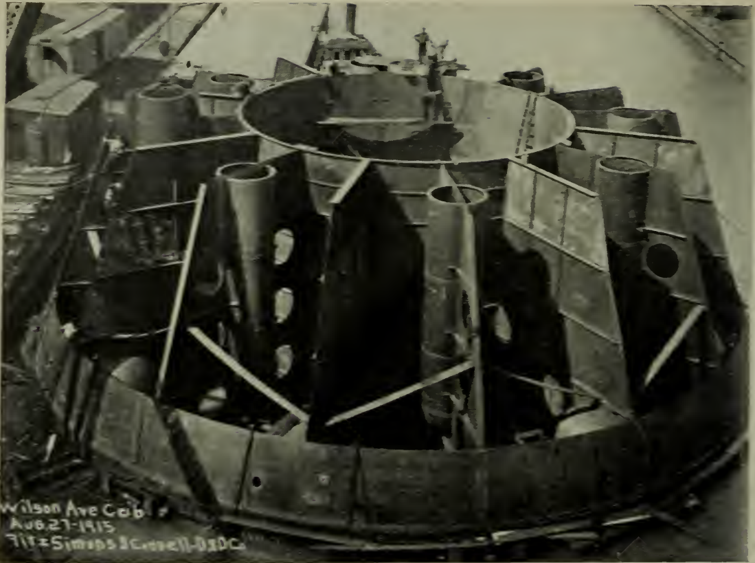
Lower Section of Steel Shell of Wilson Avenue Crib showing Buoyancy Chamber.
